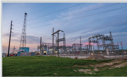
Liquid Fuel 44 MW
